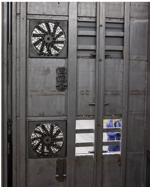
Image 44: Forced ventilation system with temperatures sensors
